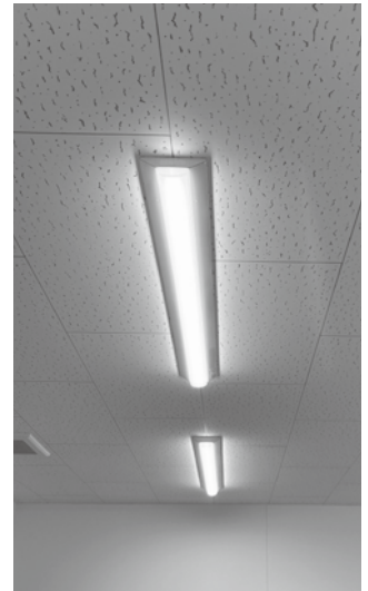
LED 照明設備
